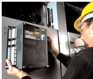
Figure 12. Permanently installed full disclosure power monitor.
